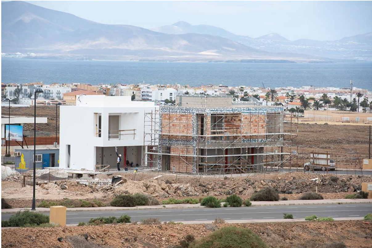
Works on a villa in the Panorama Tres Islas urbanization, in Corralejo. Photo: Carlos de Saá.
